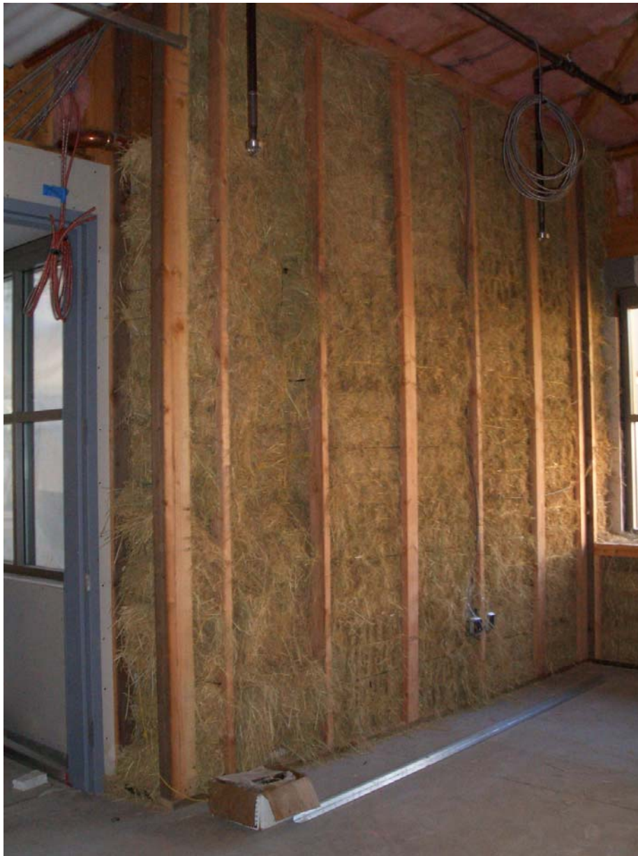
Walls in Kennedy Commons insulated with staw bales, as seen during construction
